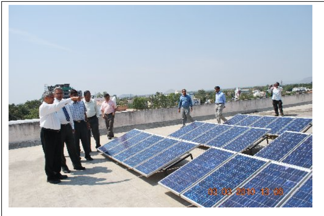
Solar panel Tribid System- Renewable Energy
